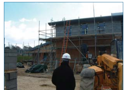
The New Music School at Reigate Grammar School – on the way towards completion for this coming July.
